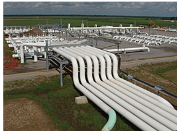
A liquid distribution manifold system at the James Terminal.
