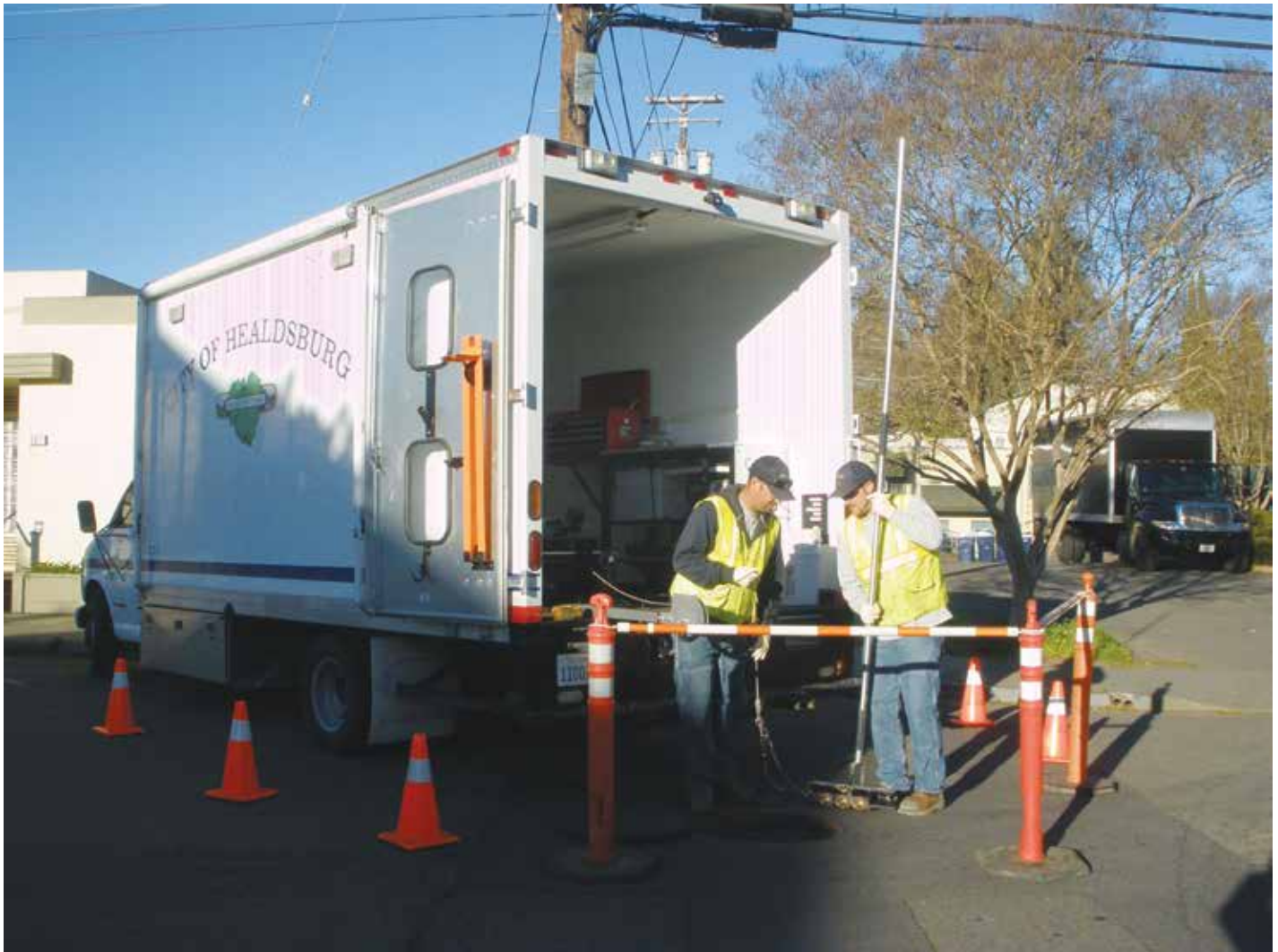
↑ Healdsburg Utilities Department staff keep the wastewater and stormwater pipeline systems in top condition. (Photo courtesy of City of Healdsburg.)
