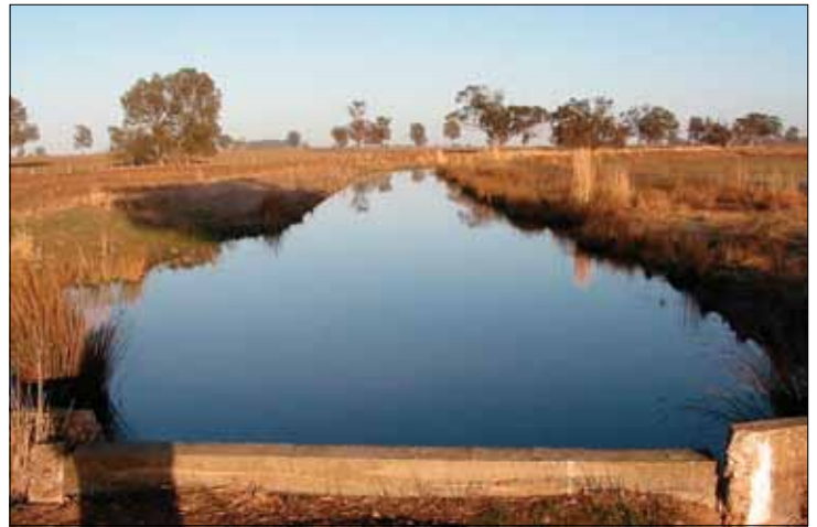
The Wimmera Mallee open-channel system was losing drastic amounts of water due to evaporation and leakage.
